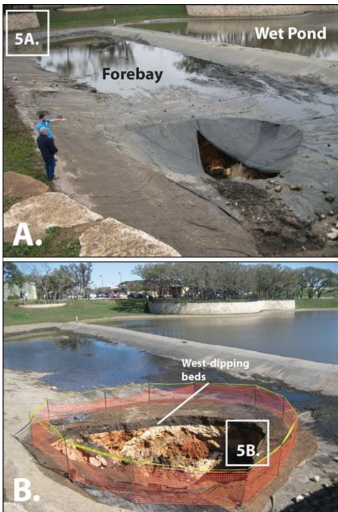
Figure 4. Photograph of sinkhole, all photos facing north. A) photo taken the day the sinkhole was observed (credit Heather Beatty, TCEQ). B) Photo taken two days after collapse and prior to excavation. Note the limestone beds are dipping to the west.
