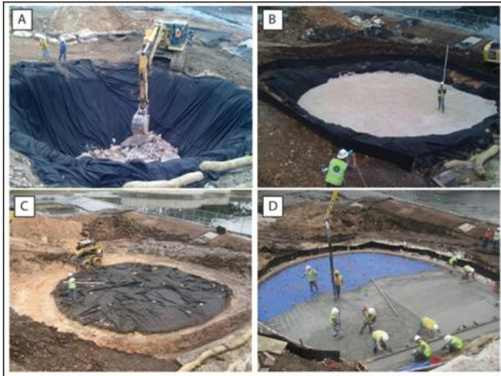
Figure 10. Photographs during sinkhole mitigation. A) Boulders and coarse fill and filter fabric; 5/2/12, B) graded cobble to gravel fill; 5/7/12, C) Gravel-filled sinkhole and filter fabric; 5/9/12, D) Reinforced concrete cap and blue vapor barrier; 5/10/12.
