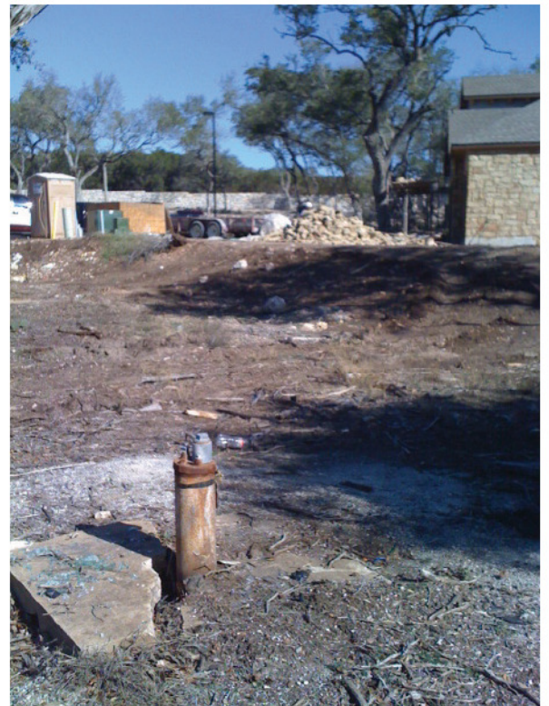
An unprotected, abandoned well with a cracked well head slab in a construction zone.
