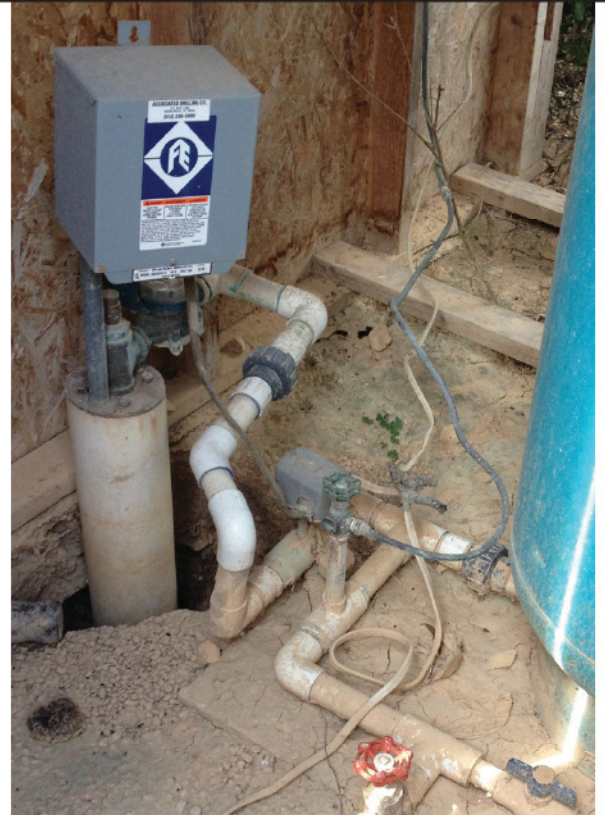
A deteriorated annular seal around a well casing.
