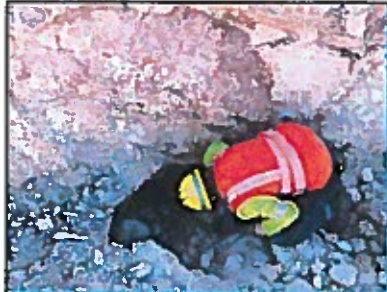
Void in side of wall for highway construction
